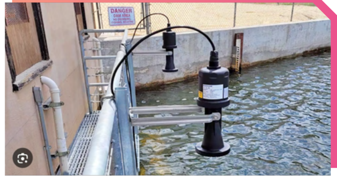
Water Level Sensors
